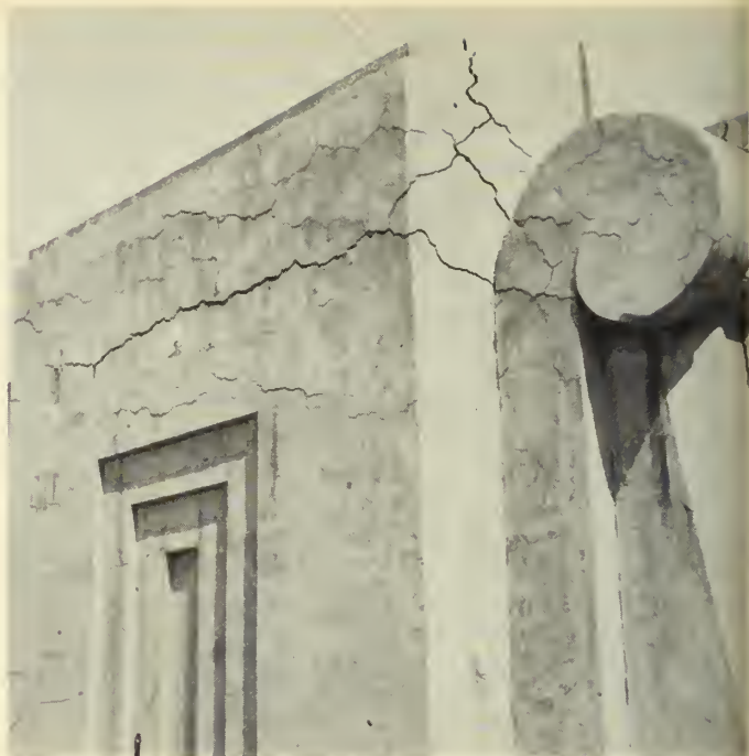
FIGURE 6. Pattern cracking in pier, Sixth Street Bridge, Los Angeles.
